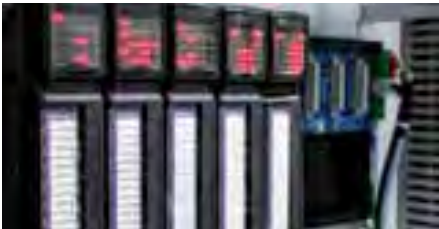
Connections to PLC
