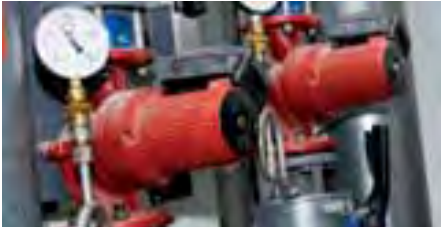
Actuators, valves, control cabinets
