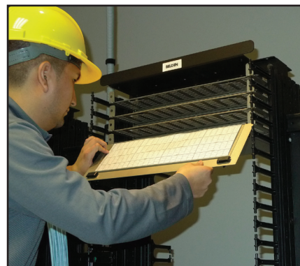
Shelf identification labeling is clearly visible.
