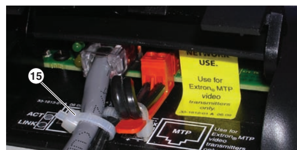
Figure 6. Securing all cables
