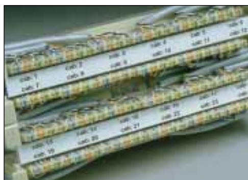
Network Systems Labeling
