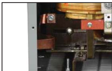
Factory installed main grounding lugs
